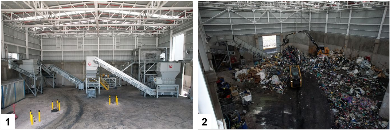
Figure 35: RDF pre-processing plant, 1) interior view, 2) plant in operating conditions, San Luis Potosí, Mexico [78]
