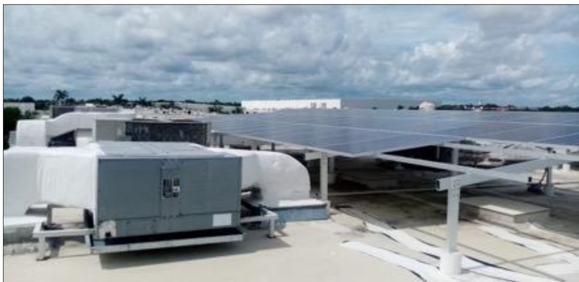
Figure 2. Project components installed on roofs or rooftops of buildings.
